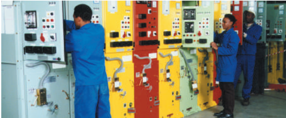
Medium voltage switchboard undergoing preparations for acceptance testing.
