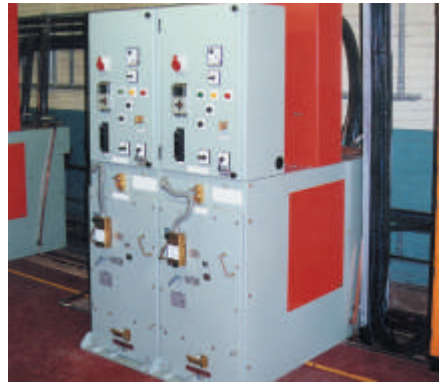
Freestanding SBV 5 capacitor feeders.
