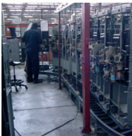
A switchgear unit being tested, making sure it complies to customer specifications..
