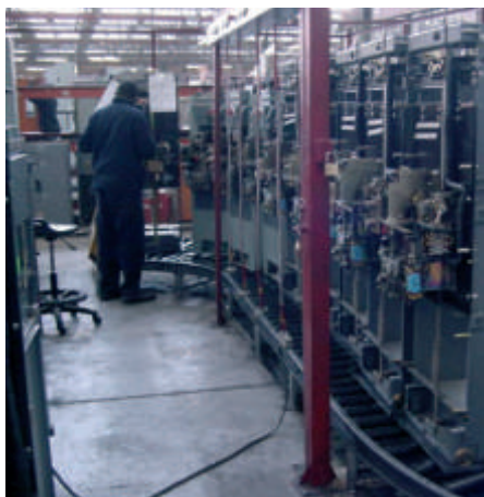
A switchgear unit being tested, making sure it complies to customer specifications..
