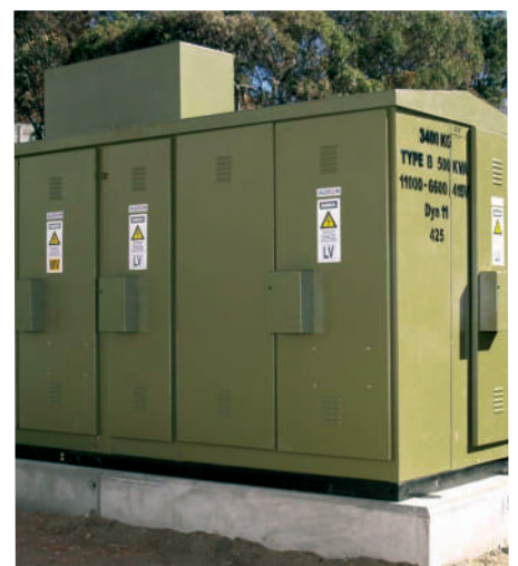
Miniature substation with IAC.
