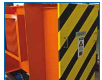
Figure 7, MV cable box IP 54
