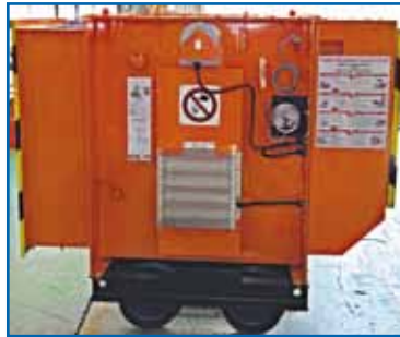
Figure 1, typical 250kVA mobile minisub
