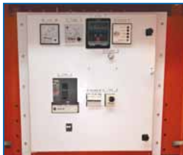
Figure 4, typical 400v LV panel
