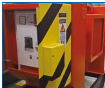
Figure 6, LV panel IP 54 rating
