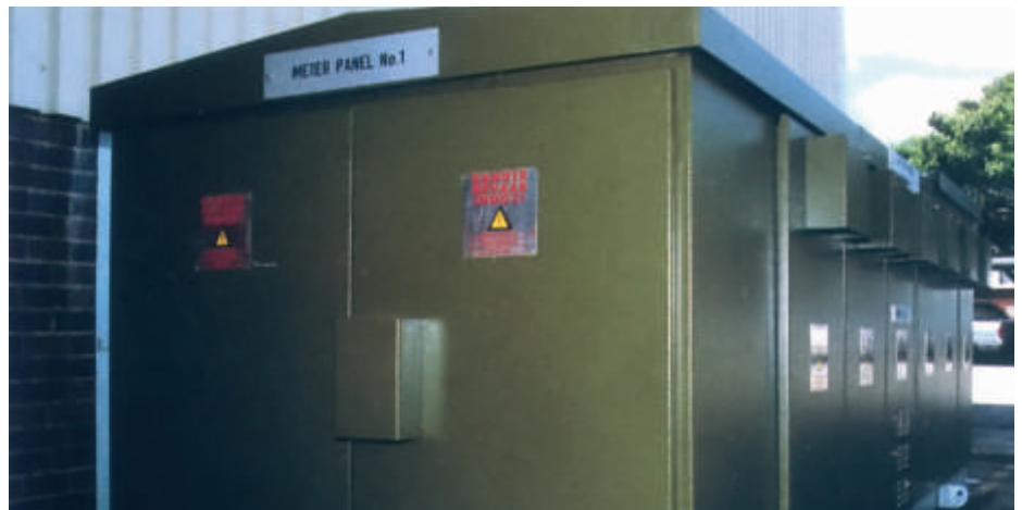
Rhino outdoor substation.
