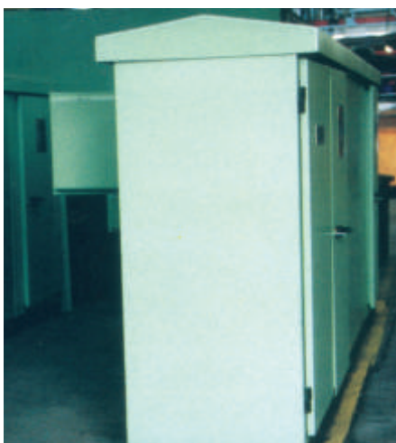
Side view of a type A miniature substation.
