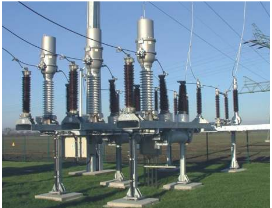
Compact air insulated switchgear (CAIS).
