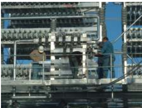
Series capacitor banks at Luckhoff.
