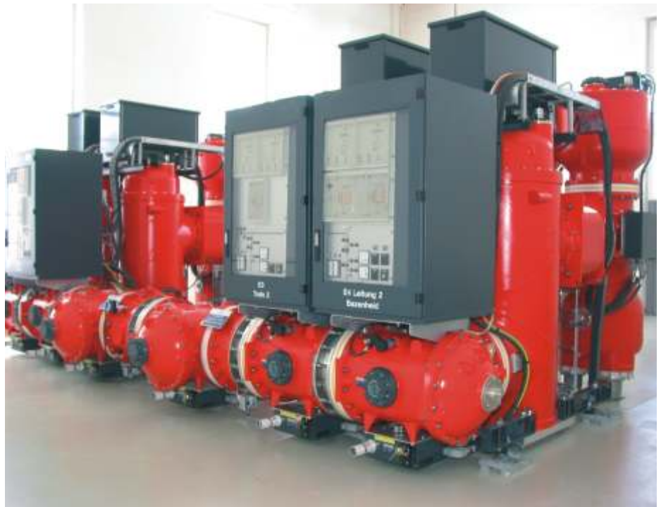
Gas insulated switchgear (GIS).
