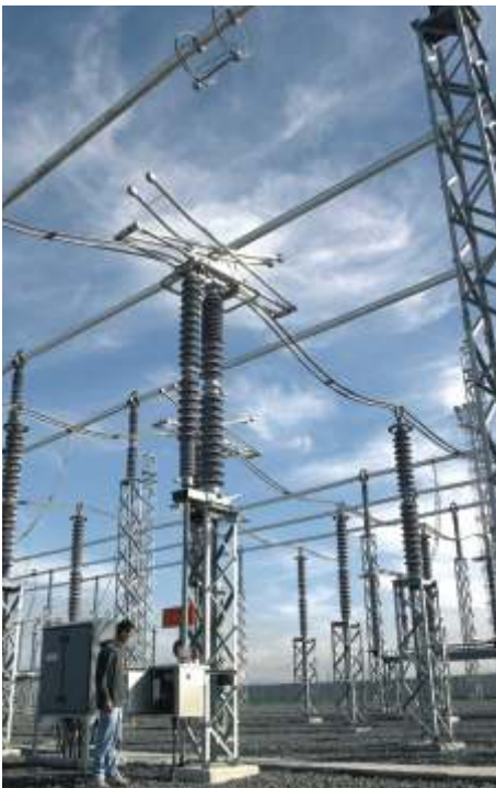
Installed pantograph isolator.
